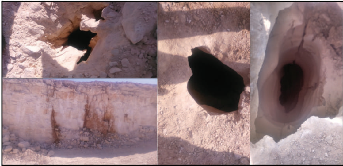
Figure 1. Examples of founded caverns that were uncovered on the construction site during excavation.
