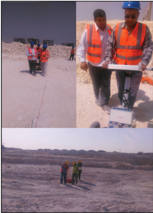
Figure 5. The GPR scan with SIR 4000 and Mala systems using 200 and 250 MHz antennas during acquisition.
